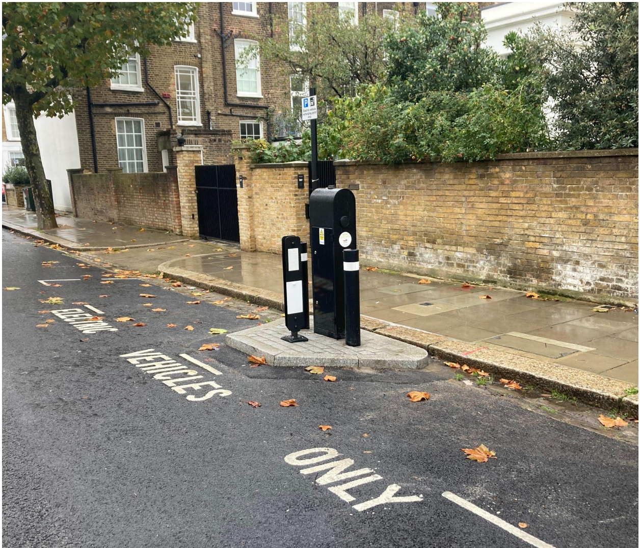
Figure 2: Example of a kerb build-out EV charging point installed in a parking bay in Camden. Credit: Possible
